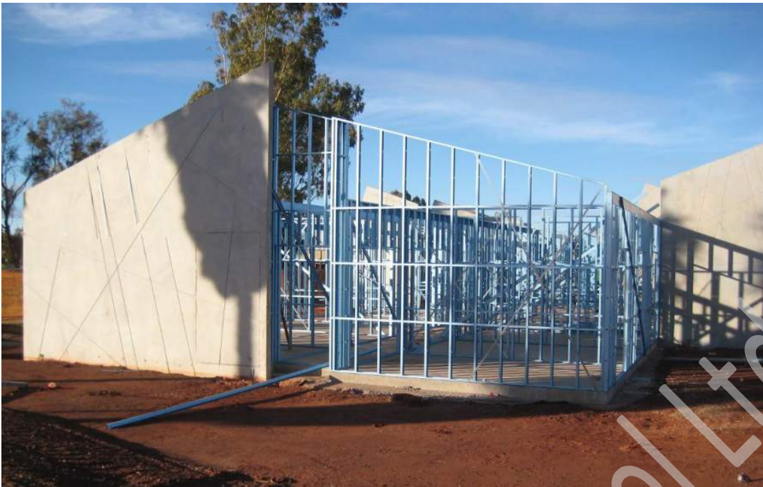
Figure 7.14 End wall placed into position and temporarily braced using clamps and/or TOPSPAN battens.
