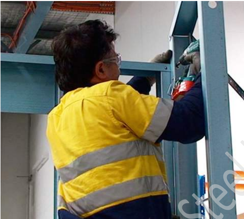
Figure 7.27 Once the frame is plumb and square, fix at the top of the wall.
