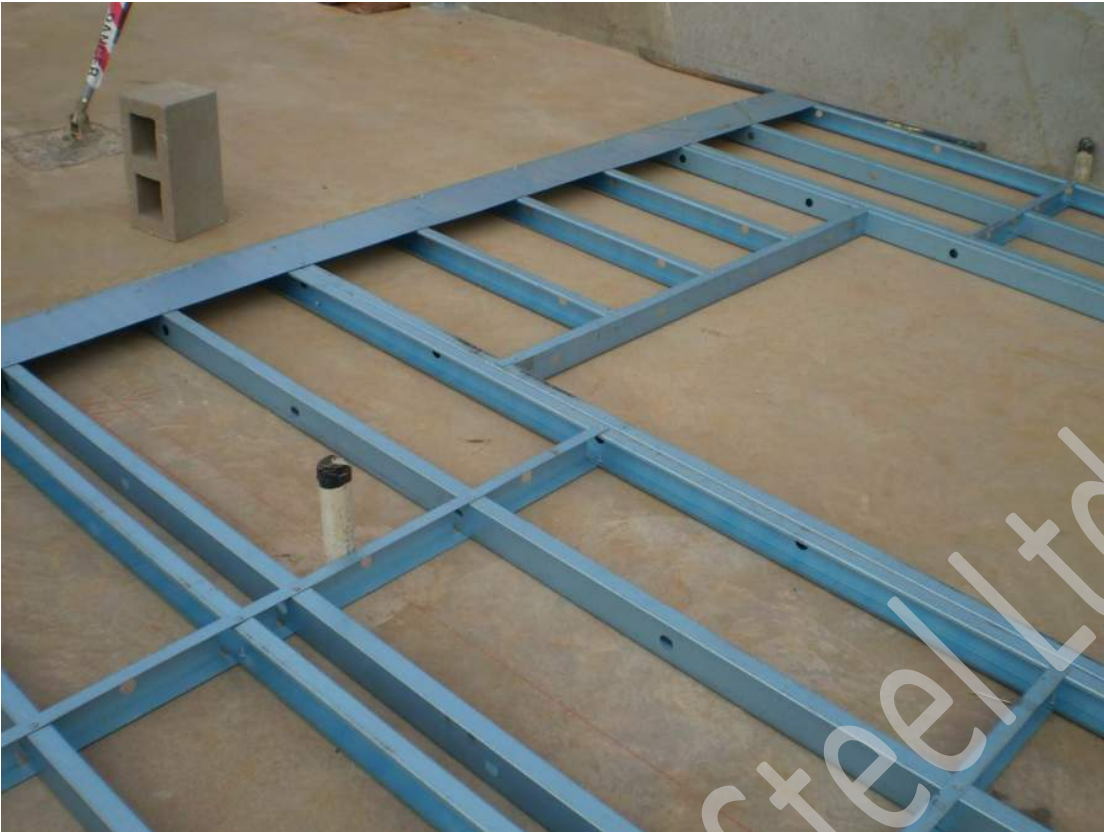
Completed wall frames to be stacked in a flat area ready for installation.
