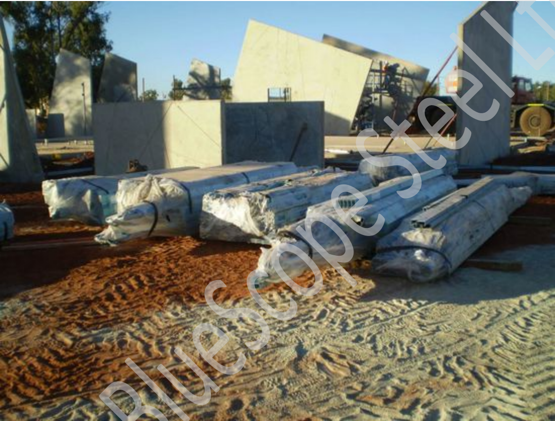
Wall & truss framing will be plastic wrapped & labelled in bundles as registered on packing list
