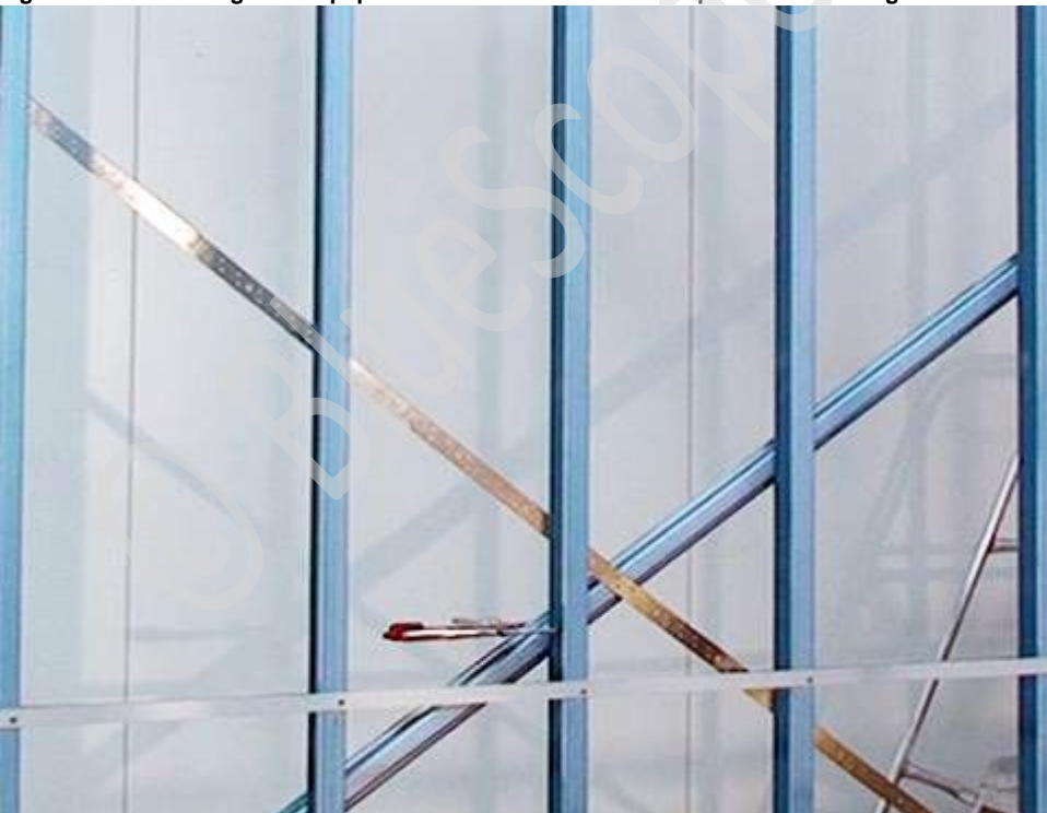
Figure 7.28 Use strap bracing and tensioner to set frame square and plumb. Note vice grips at mid-span.
