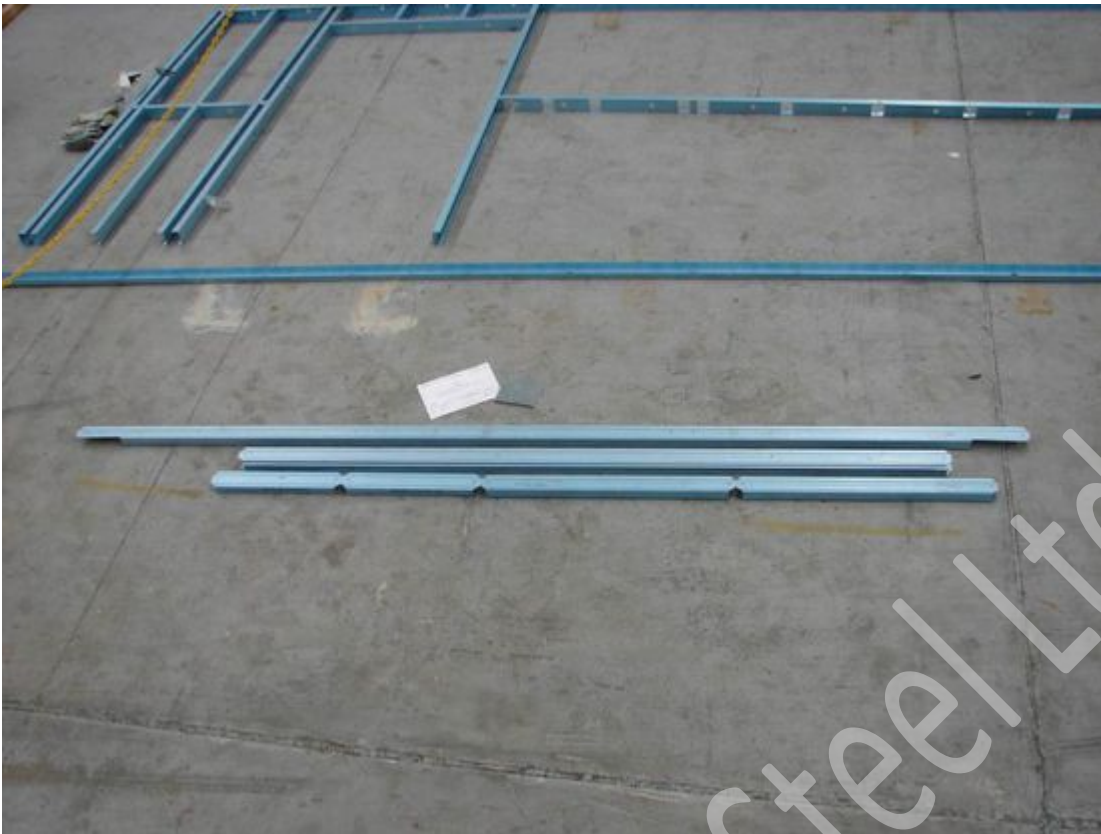
Separate and move stud & nogging / plate frame packs next to designated assembly zone.
