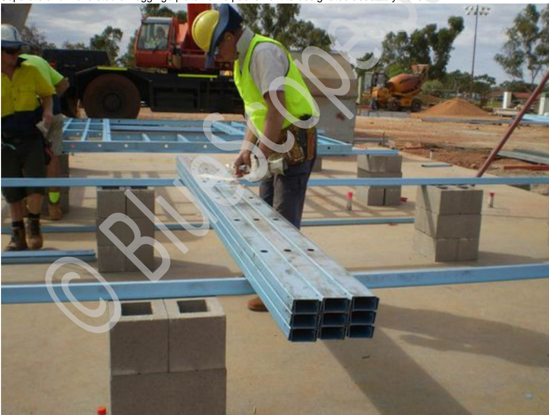
Lift & separate stud pack onto assembly table (this example has utilised Topspan ® 40 sections on concrete block stacks as an assembly table).
