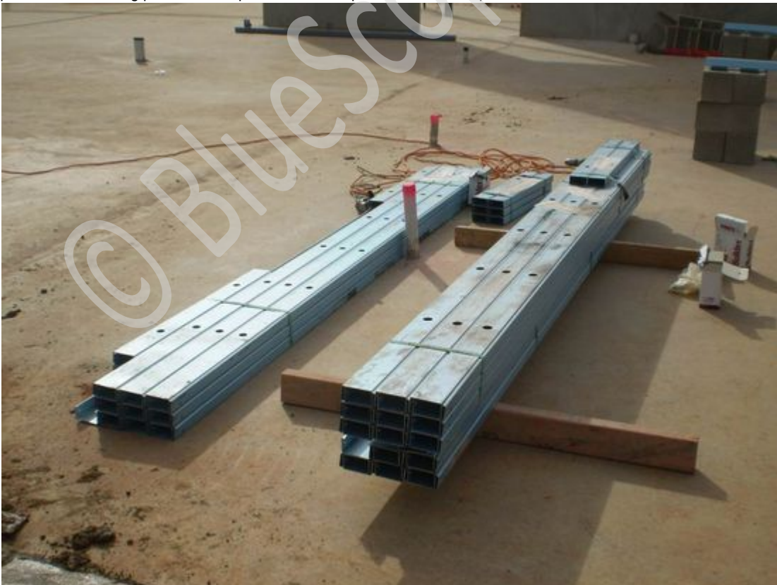
Locate & open matching stud & nogging / plate bundles before separating into individual frame packs.
