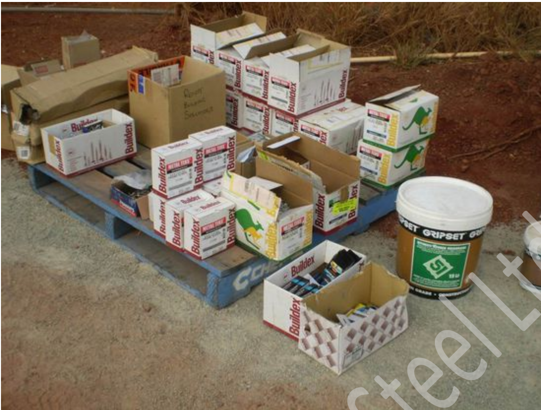
Sort & stack all accessories, cross check packing list. (helps to mark on box's, where accessories are to be used)
