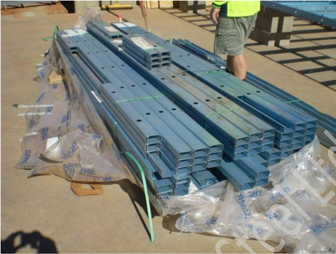
Wall frames are individually strapped & stacked in "stud" bundles, labelled with bundle numbers
