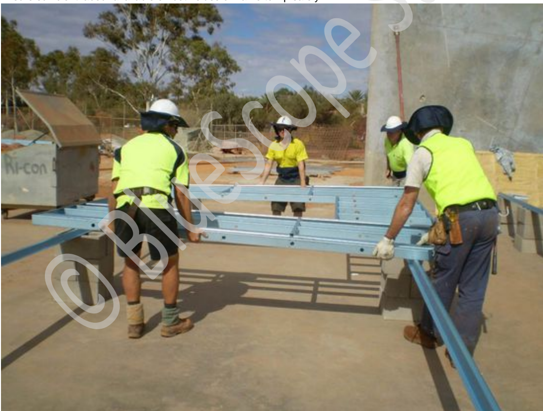
By utilizing two adjoining assembly tables, wall fabrication can be optimized by preparing the next frame while screw fixing & checking "Side B".
