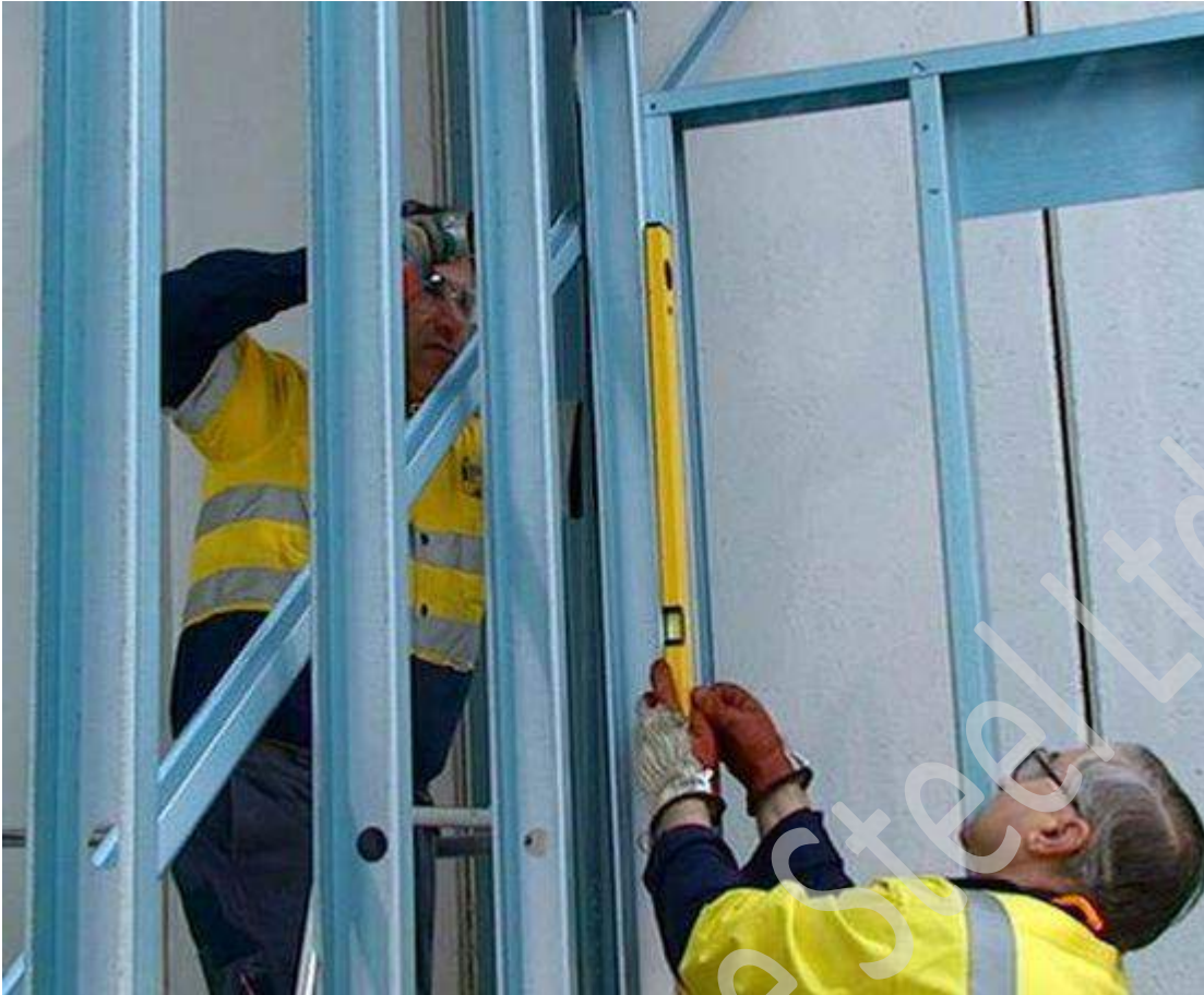
Figure 7.26 Use a length of Topspan batten to hold the frame square until bracing can be tensioned.
