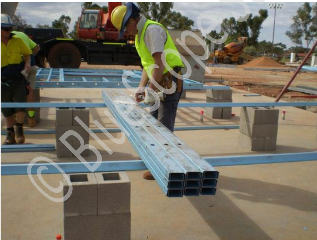
Lift and separate stud pack onto assembly table (this example has utilised Topspan® 40 sections on concrete block stacks as an assembly table).
