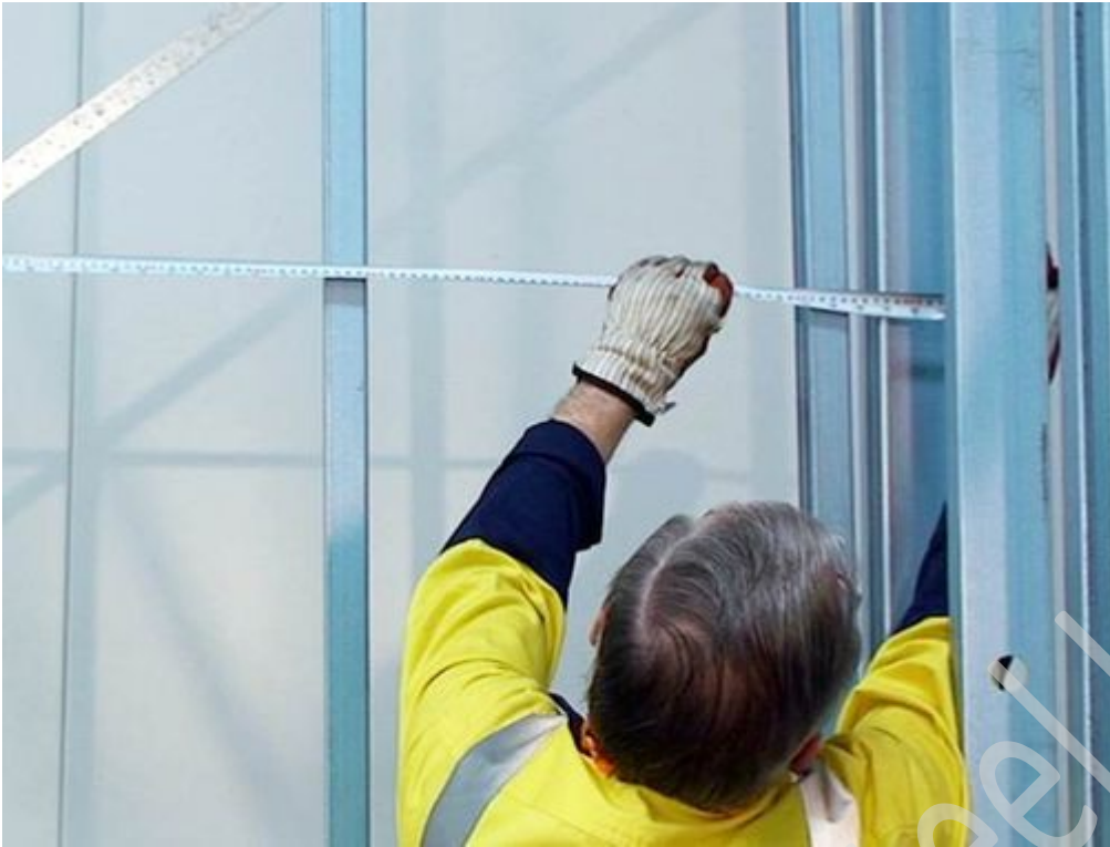
Figure 7.22 Measure lengths at bottom and top of wall to check frame is square.
