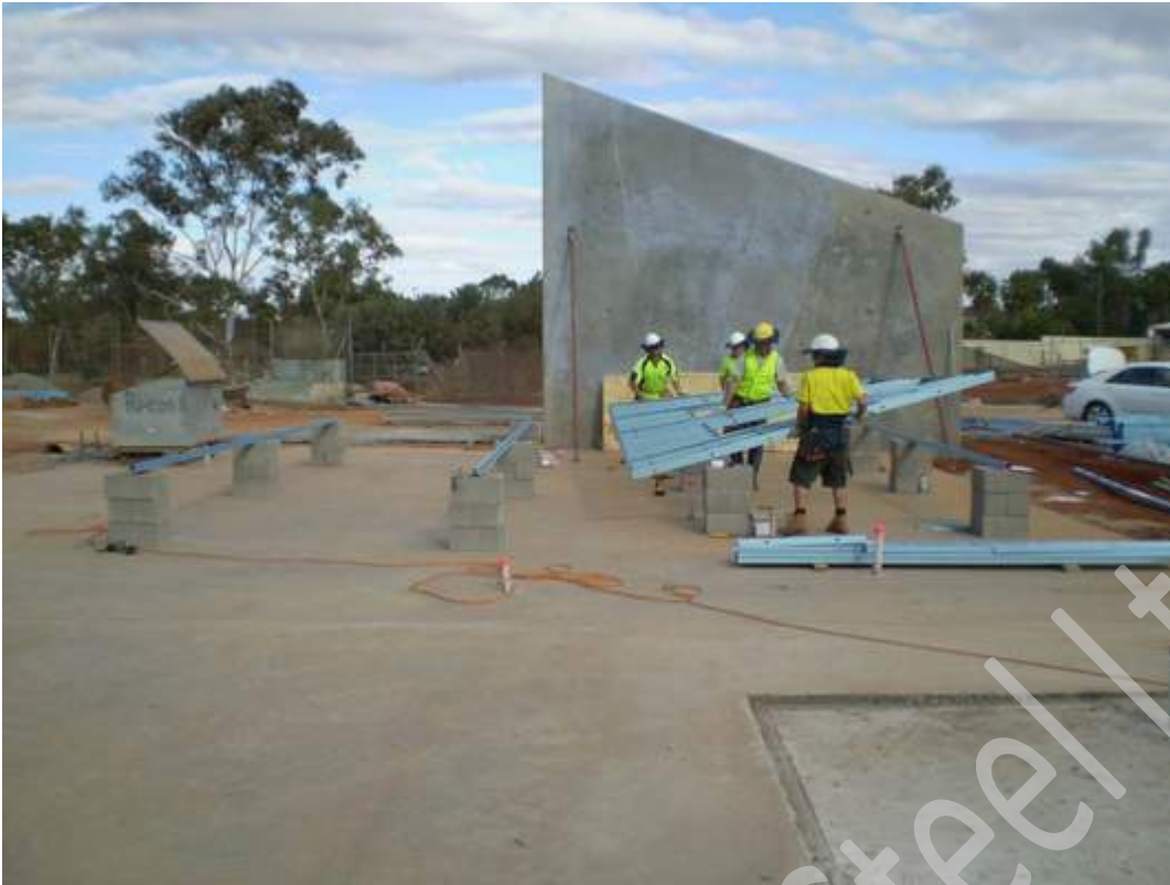
Cross check "Side A" frame layout & connections as per assembly sheet. Utilizing sufficient labour, lift & flip frame for "Side B" screw fixings.
