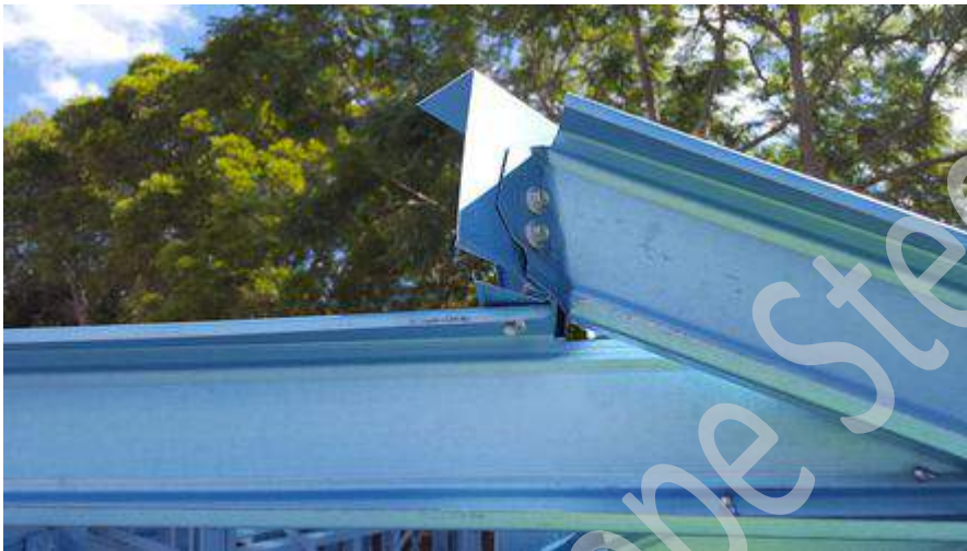
Figure 7.35 Veed hip rafter connecting to first station truncated truss (note: bottom flange of vee hip plate notched)
